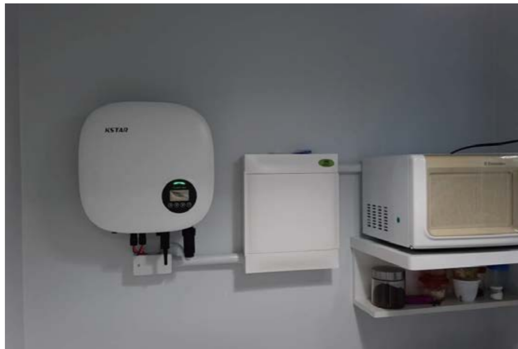
03 Residential Solar Project in Brazil
