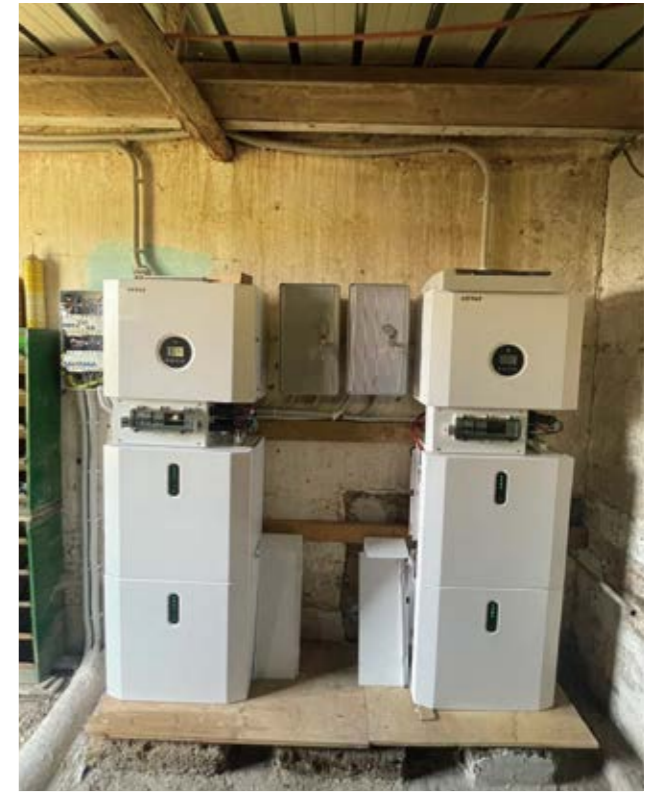
08 Residential ESS Project in Italy
