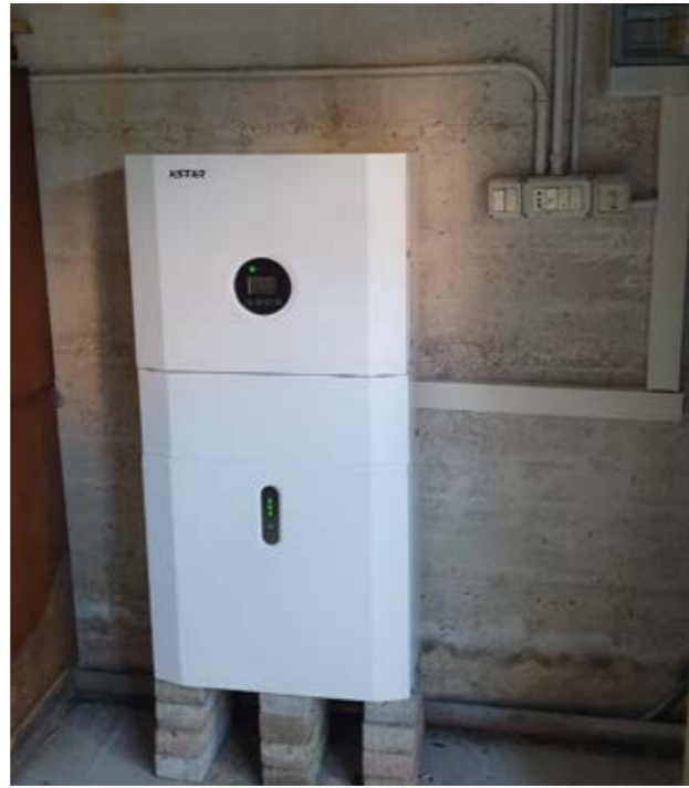
06 Residential ESS Project in Italy
