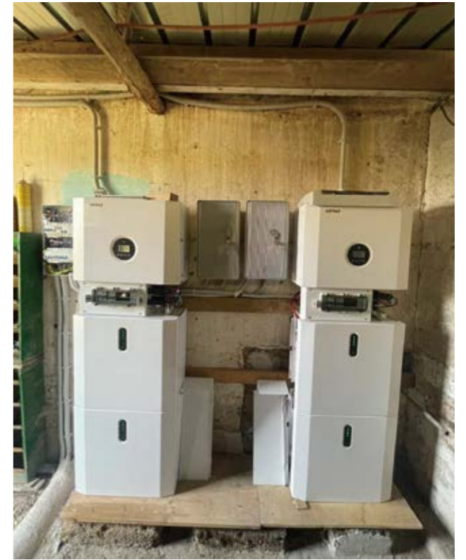
08 Residential ESS Project in Italy
