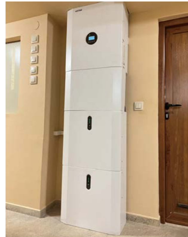
10 Residential ESS Project in Bulgaria
