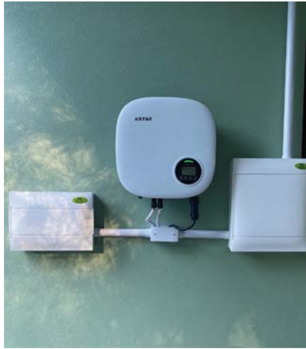
05 Residential Solar Project in Brazil
