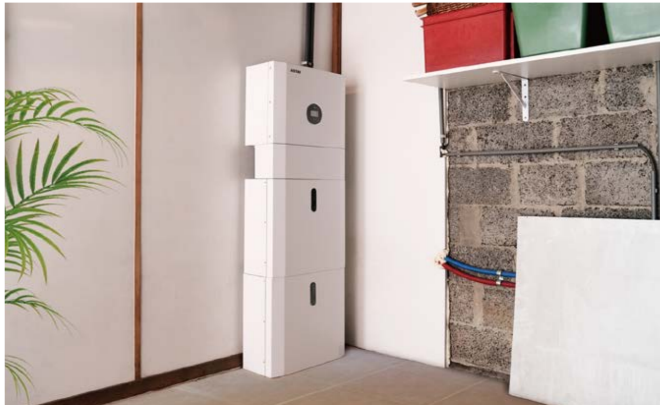
09 Residential ESS Project in the Netherlands
