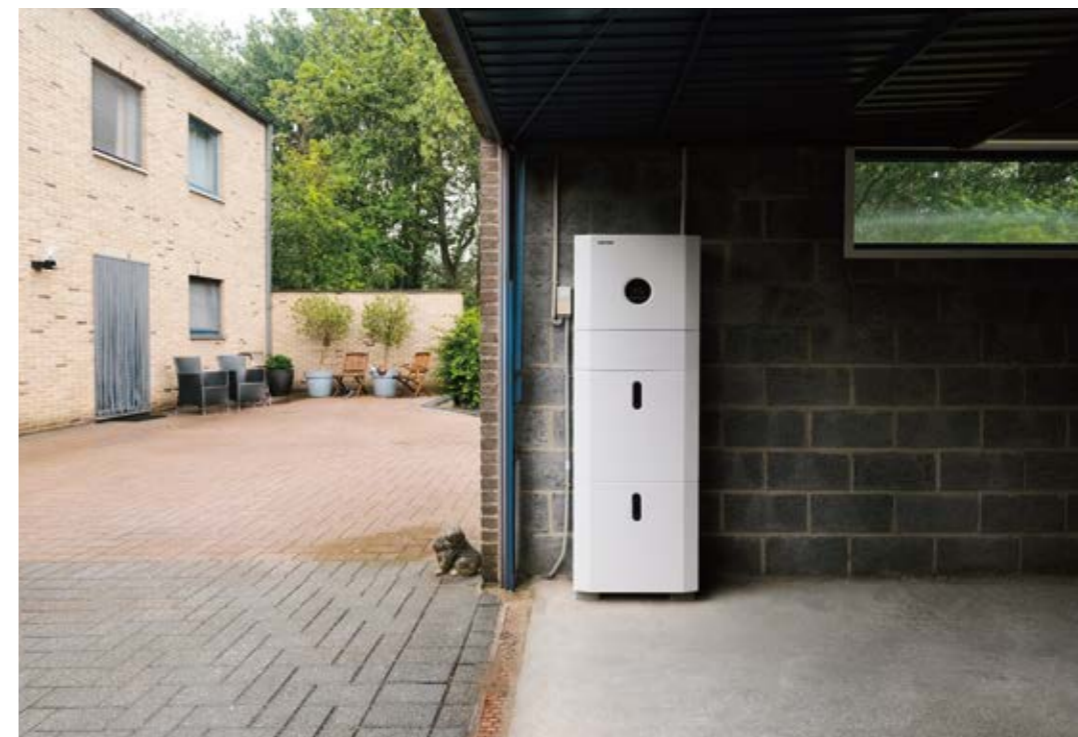
04 Residential ESS Project in Belgium
